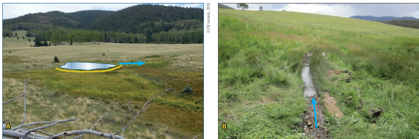
Figure 4.16A. The photograph shows a nonfunctioning stock pond with a breached berm in Middle Holman Creek. Figure 4.16B. The breach was plugged and a treatment train was installed at the pond spillway to send water to drying wetland on valley right. Blue arrows indicate flow path.
