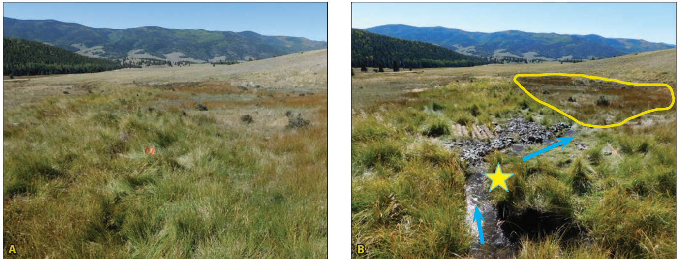
Figure 3.4A. Photograph faces downvalley in East Holman Creek before structures were built to stabilize a headcut (orange flags). Figure 3.4B. The constructed keypoint (yellow star) holds and directs water across the landscape dissecting the stream's flow to a drying wetland (evidenced by Juncus rather than Carex vegetation). The yellow polygon indicates target area of Juncus for re-wetting. Blue arrows indicate flow path.
