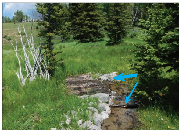
Figure 4.1. A log step fall to stabilize a headcut is elevated to split channel flow to a lead-out berm. The lead-out berm was excavated a few inches deep to achieve a suitable elevation for capturing and directing the flow that was split from the main channel. Blue arrows indicate flow path.
